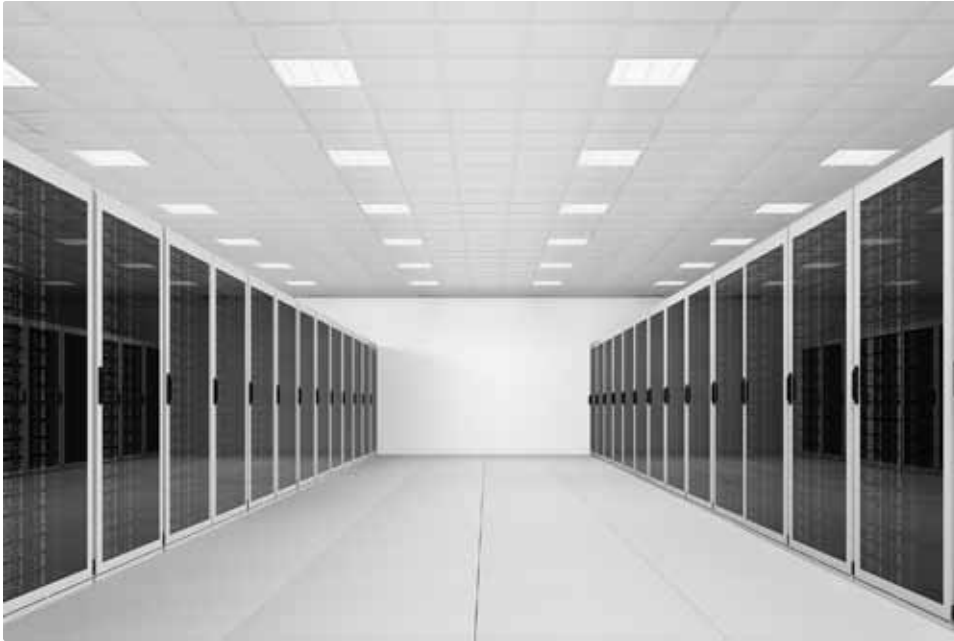
FIGURE P13.1 A server farm.
